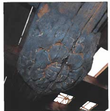
Charred surface of a boss from the ceiling of the nave
