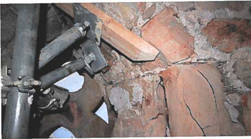
Cracked and spalling masonry in the tower caused by the cooling effects of water from the fire hoses when fighting the fire
