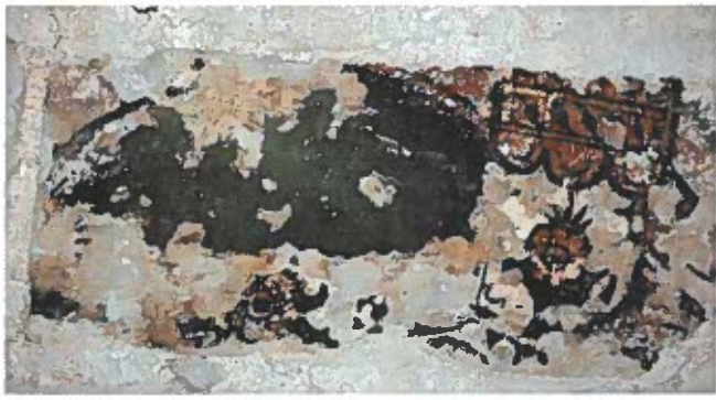
Painted decoration from the late 15th or early 16th century which was uncovered during the work
