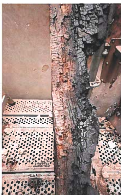
Not all the roof timbers could be salvaged.
