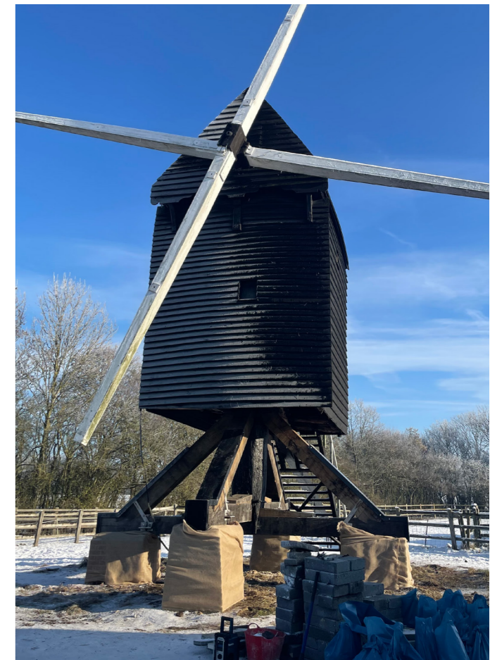
▼▼ Figure 7 - Scaffolding down and hessian wrapped around rebuilt brick piers to protect from frost as the mill nears the end of its restoration
